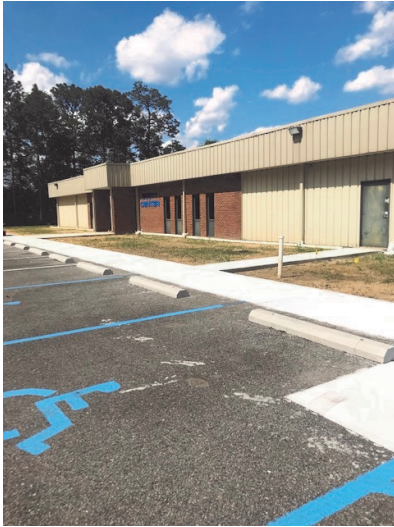
Repaired Gutter System and Landscape to keep water from flowing into the building
